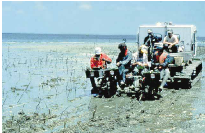
Marsh planting: Effective contract specifications are necessary for successful marsh planting operations
